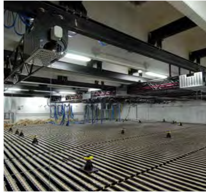
Movable stage hoists with variable speed (Load: 1.000 kg)
