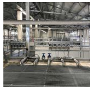
Depuratore Falcade, piping
